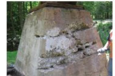
Fig. 4.1.4a—Trestle of the railway bridge before repair
